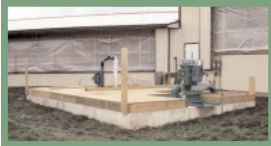
Manure Collection Pumps and Reception Pit
