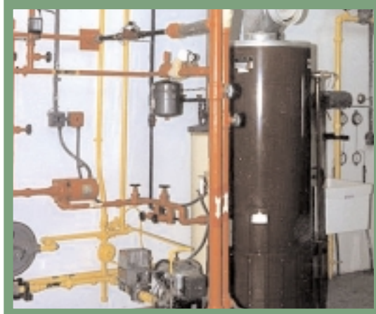
Hot Water Heater and Controls
